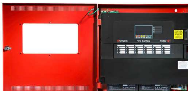
Fig 1: 4007ES panel inside view
